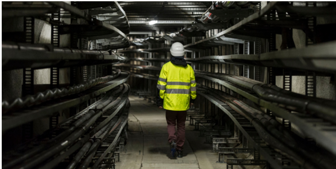
Example of cabling in a tunnel
