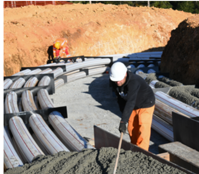
Example of cabling in a cable conduit block
